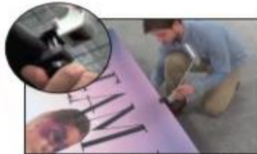
Add lighting. Tighten clamp on lighting.
